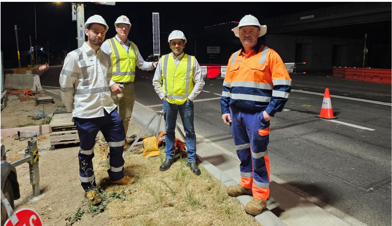
Site inspections with Transport for NSW at the Wallgrove Road in-field assessment, October 2023.
