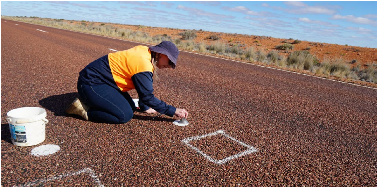
The latest inspection of sprayed seal trial sites in Coober Pedy indicate polymer modified binders are aging better than unmodified bitumen.
