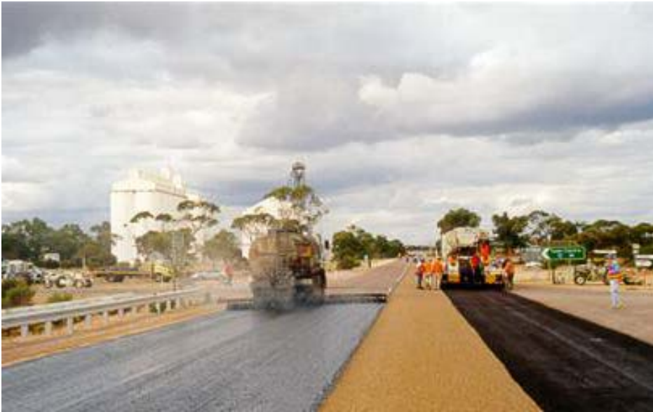
Figure 2.11: Placing cape seal showing sequence of sprayed seal binder, aggregate and application of slurry surfacing
