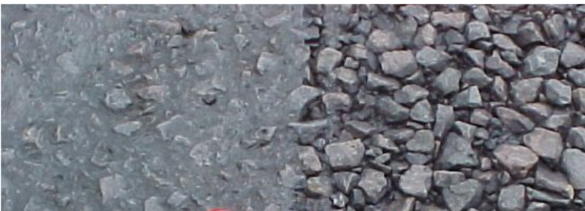
Figure 9.2: Flushed sprayed seal surface (left) treated with high pressure water (right)
