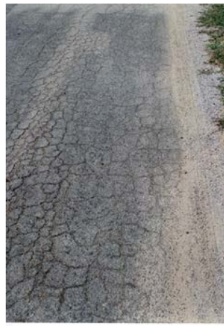
Figure 4.13: Typical crocodile cracking
