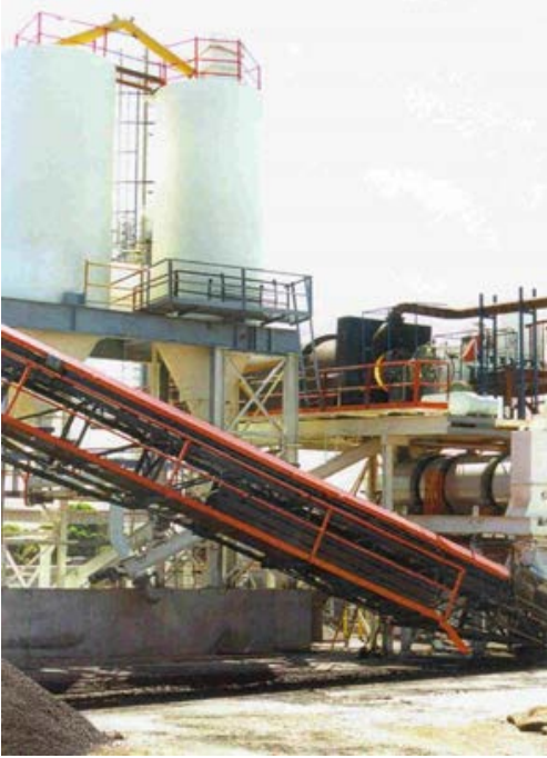
Figure 5.10: Tandem drum mixer at an asphalt plant
