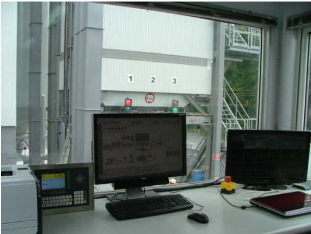
Figure 5.3: Asphalt plant control room
