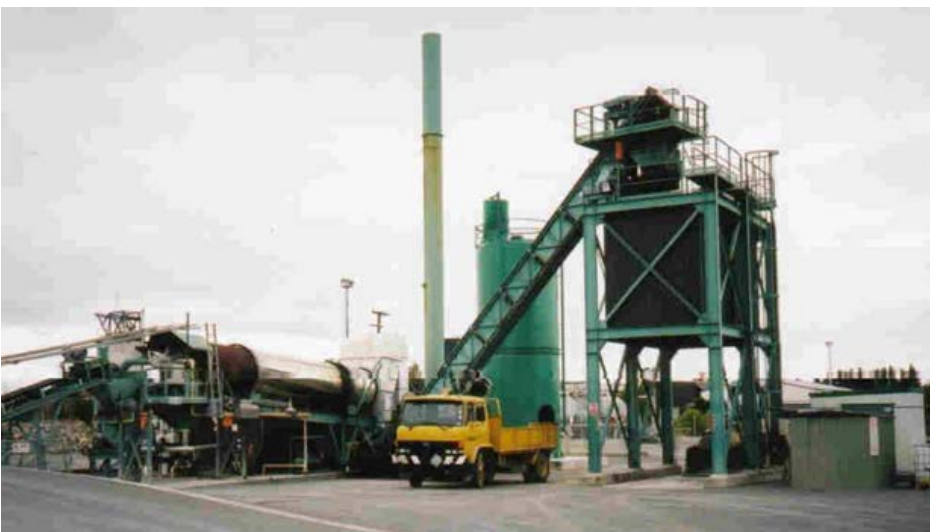
Figure 5.5: Typical parallel flow drum mixing plant
