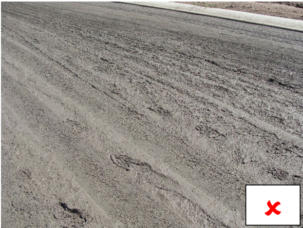
Figure A 3: Examples of poorly prepared granular pavements
