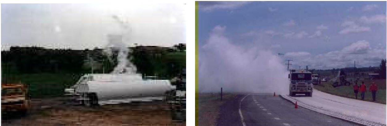
Figure 3.1: Quicklime slaking in tanker or when spread on roadway prior to mixing
