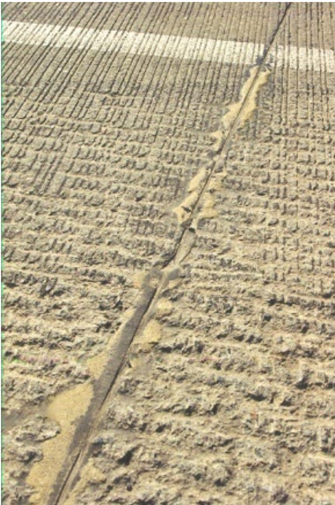
Figure 8.4: Joint damage and harsh surface texture caused by cold planing
