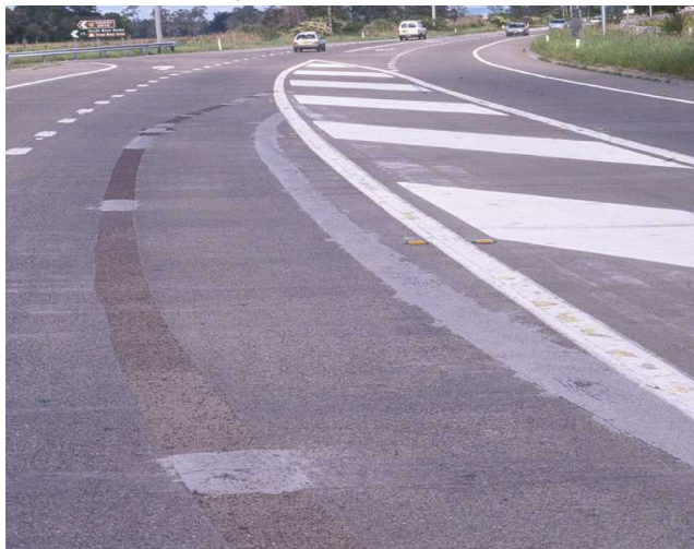
By comparison, similar repairs carried out using inferior products and/or methods have shown a high maintenance demand
