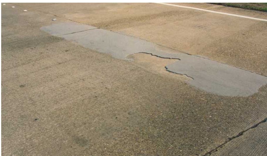
Figure 8.3: An unsuccessful thin bonded topping
