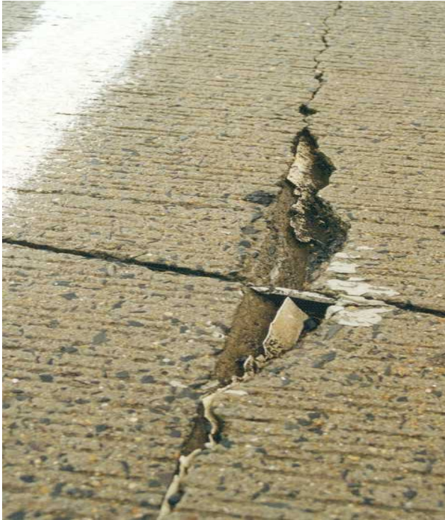
Figure 8.8: Spalling at an inclined and depressed ribbon in a longitudinal joint
