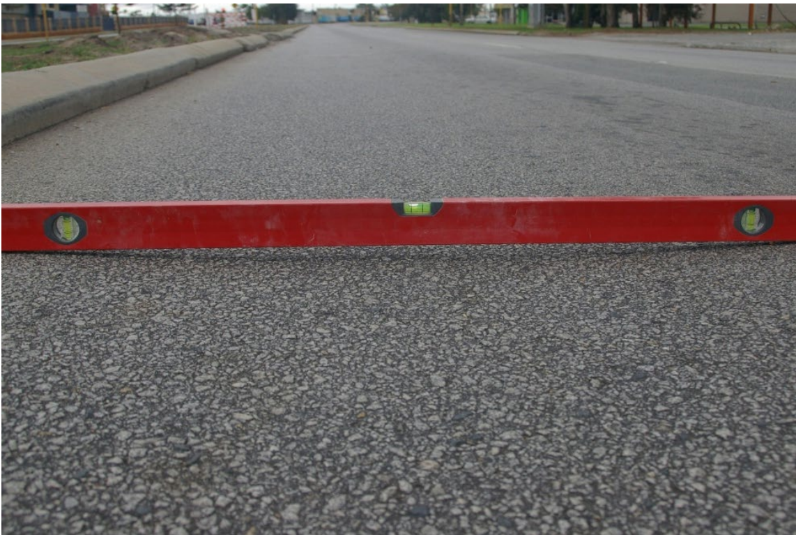
Figure 4.4: Rutting in a wheelpath
