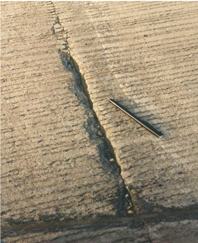
Spalling at a longitudinal tied joint
