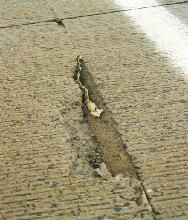
Figure 8.7: Spalling at an inclined ribbon in a longitudinal joint
