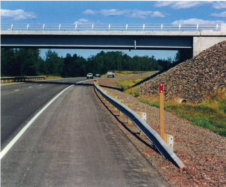
Figure 6.17: Hazardous turn-down barrier end treatment
