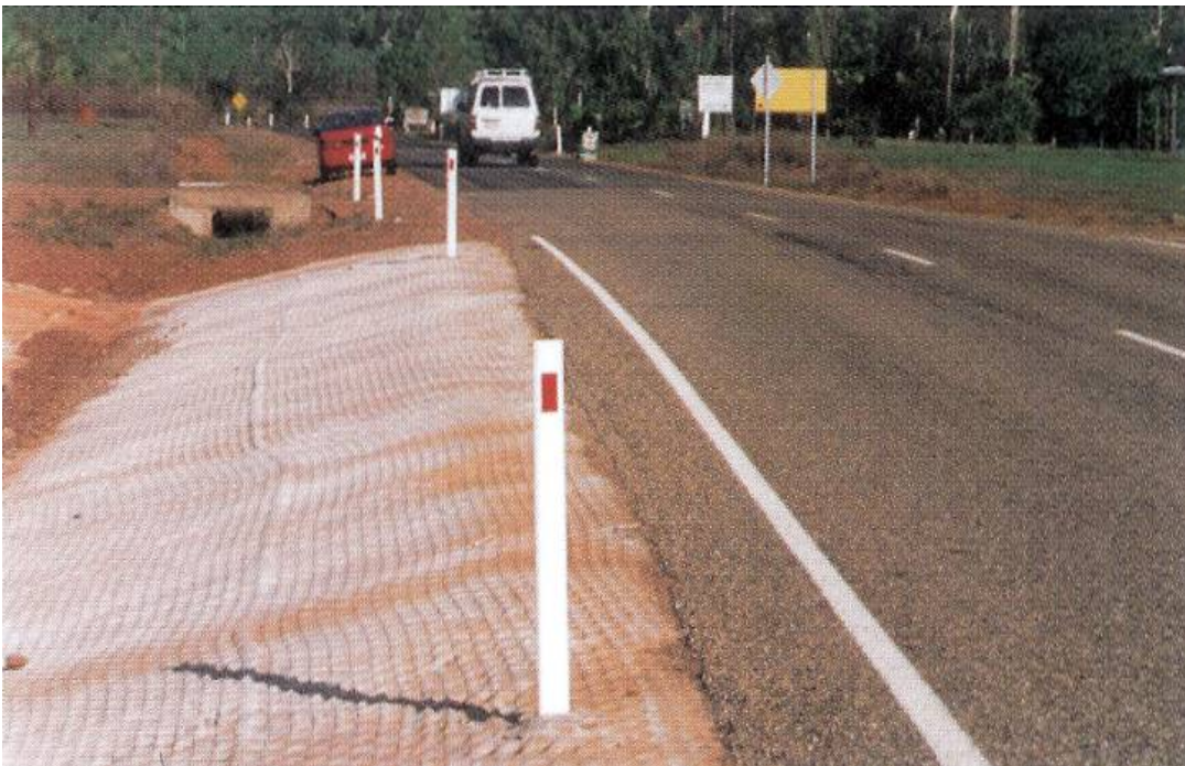
Figure 6.13: Non-traversable culvert end wall
