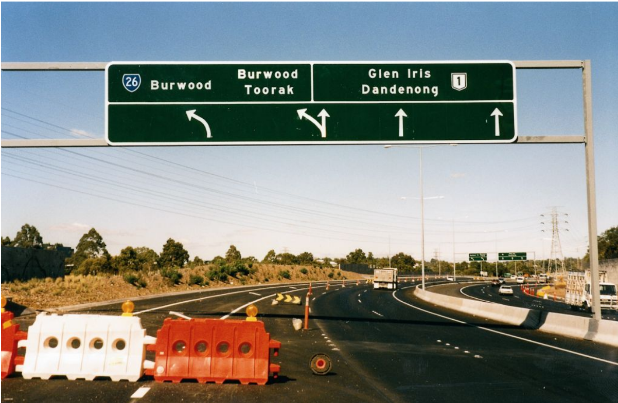
Figure 5.6: Incorrect sign installation
