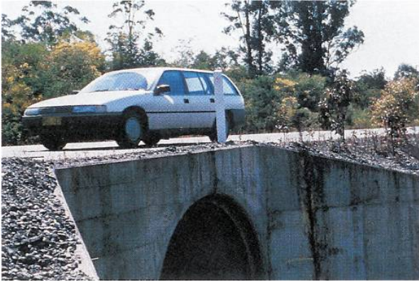
Figure 7.22: Unshielded deep drains close to the road are a hazard
