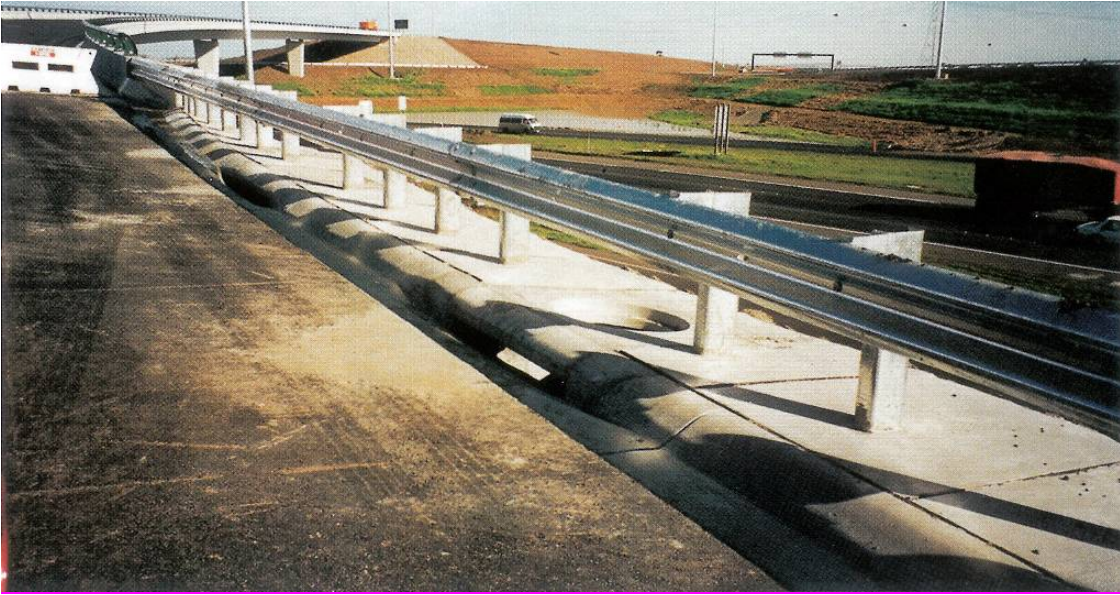
Figure 5.8: Deletion of safety barrier posts
