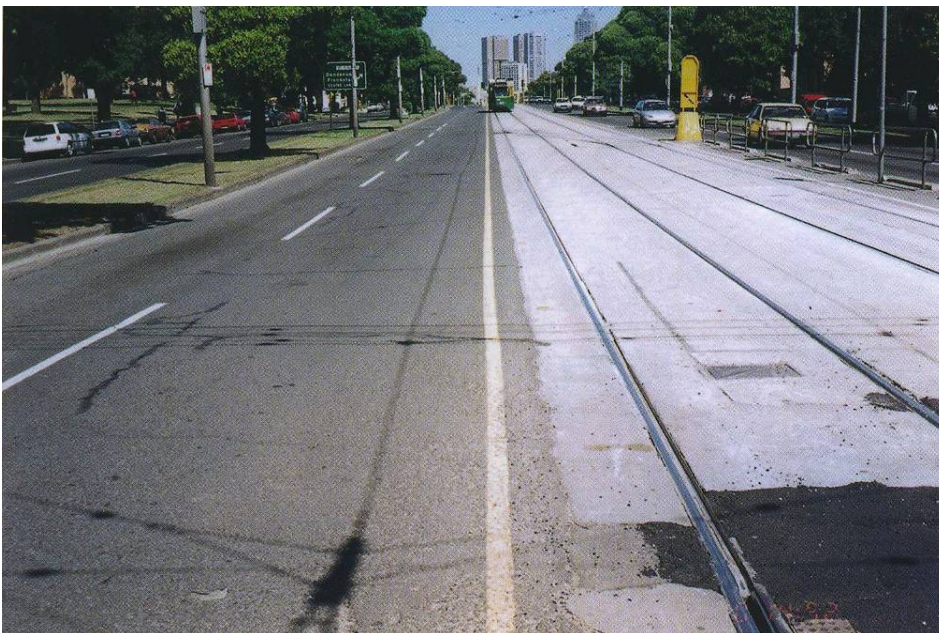
Figure 7.7: Looking south-east from the intersection to where the new refuge island will be built; poles 32 and 33 are on the left
