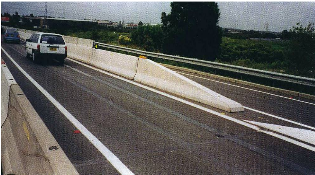
Figure 7.15: The tapered end of the concrete median barrier could result in a vehicle launching or overturning on impact
