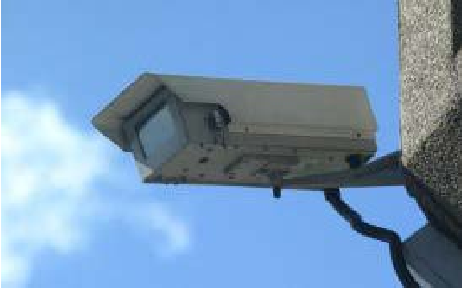
Figure 7.19: Street focused CCTV
