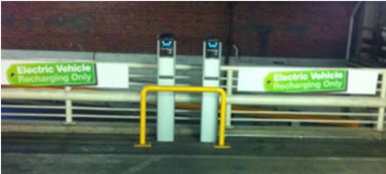
Figure 7.8: Electric vehicle charging bays – Adelaide City Council – Market Street car park
